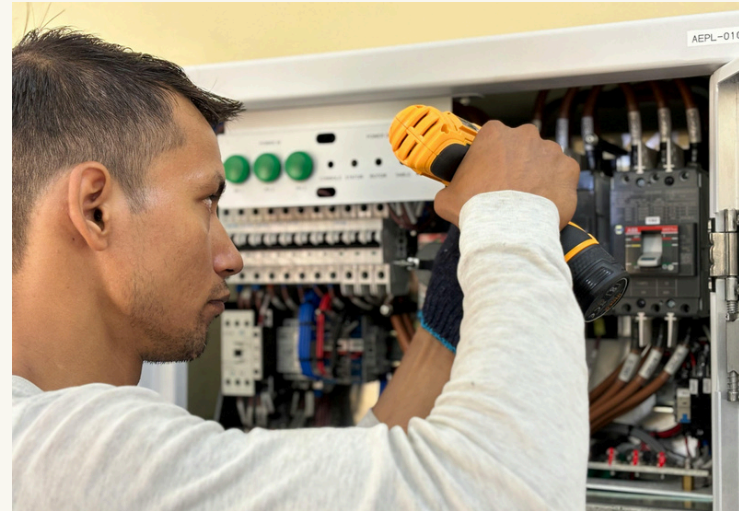
Electrical Maintenance & Wiring
